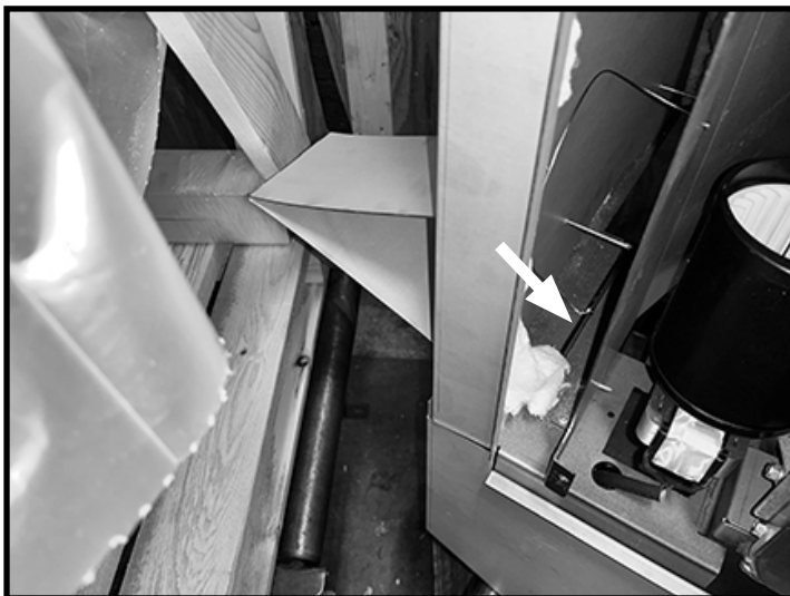
Figure 29: Rating label in place.
